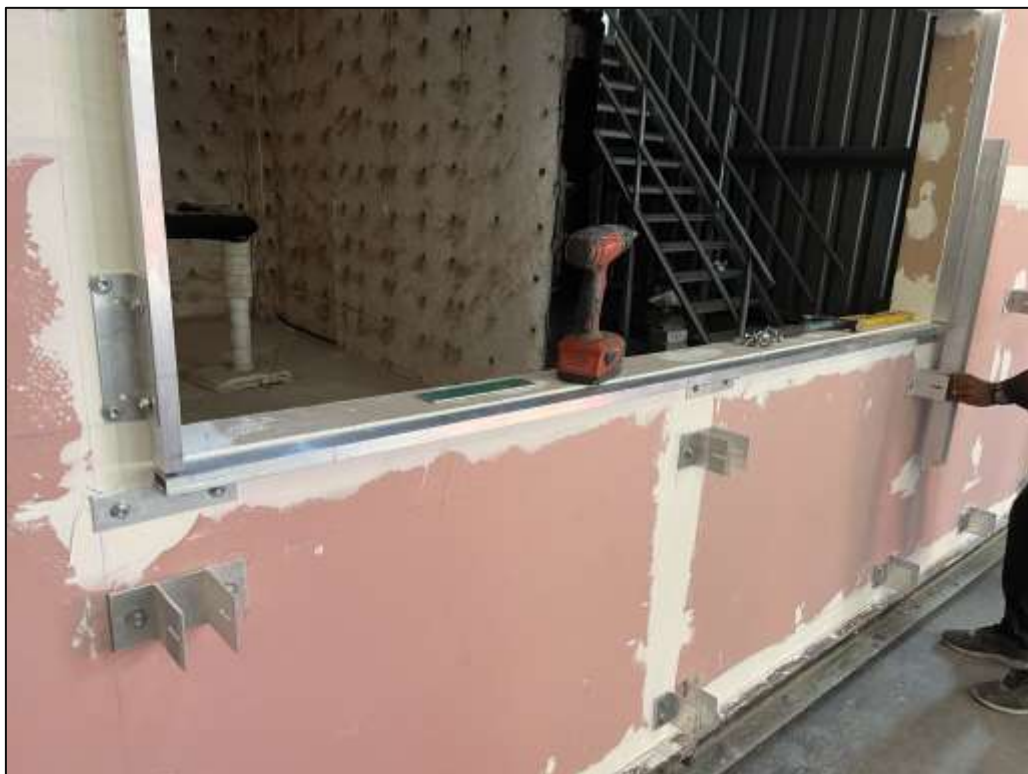
Picture 2: View of the steel tube channels fixed along the perimeter edge of the window opening.
