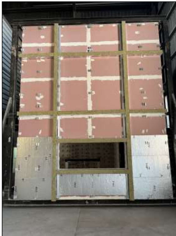
Picture 4: View of the completion of the cavity fire barriers and start of the exterior insulation.
